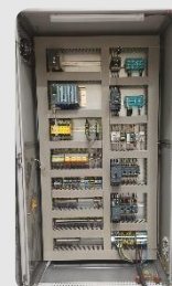
CE-Label Electrical System
