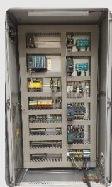
CE-Label Electrical System
