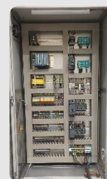
CE-Label Electrical System
