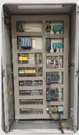
CE-Label Electrical System
