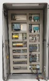
CE-Label Electrical System
