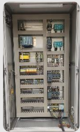
CE-Label Electrical System
